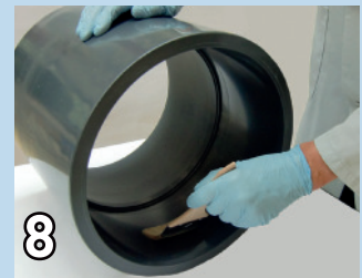
8 Apply TANGIT solvent cement centered to the fitting socket surface & distribute it first radially than axially (1 person)
