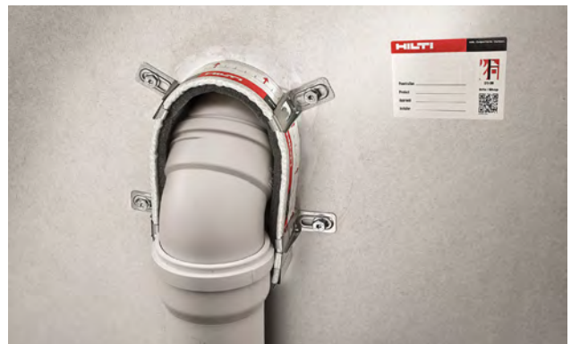
Pipe elbows in the ceiling area (2 x 45° or 87°)
